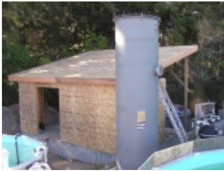
Pump / filter shed with biofilter
